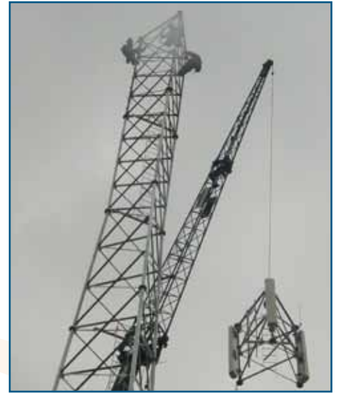
Workers assemble a cell tower near Peerless in this 2007 file photo. Cell site construction often continues into the winter months.
